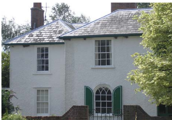
Natural slate roof, roughcast render and vertical sliding sash windows at Lascelles Lodge, Grade II listed.
