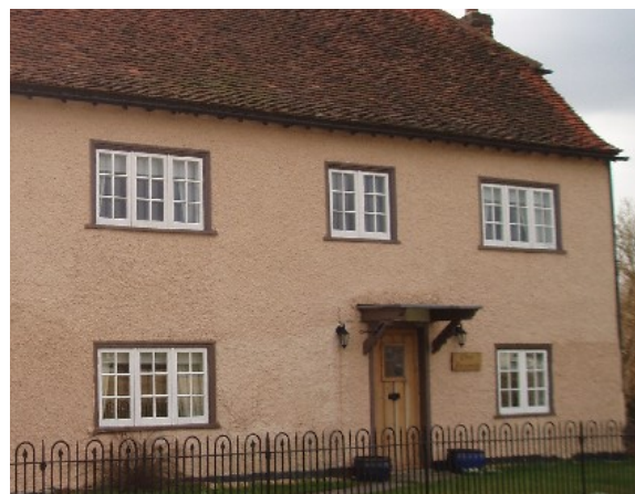
Roughcast render, side-hung timber casement windows, plain red clay tiles and traditional cast-iron railings on Elms Farmhouse, Grade II listed
