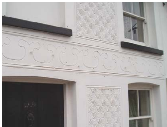
Decorative pargetting and traditional double-hung vertical sliding sash windows on the White Horse pub and restaurant, High Street
