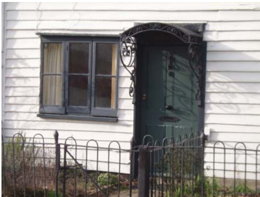
Traditional timber door and side-hung casement window and 19 th century wrought iron canopy and railings on St Anne's Cottage, Harlow Rd
