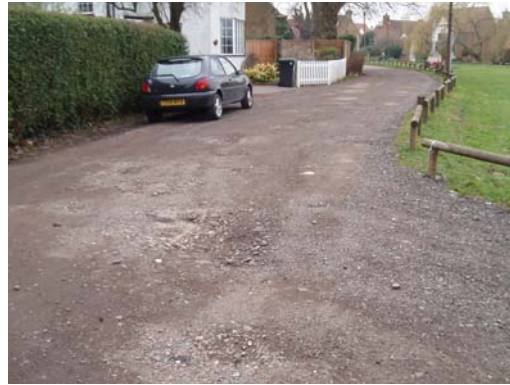
Potholes in a road around the village green
