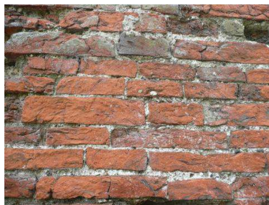
Red brick wall to Abbey Gatehouse (EFDC)
