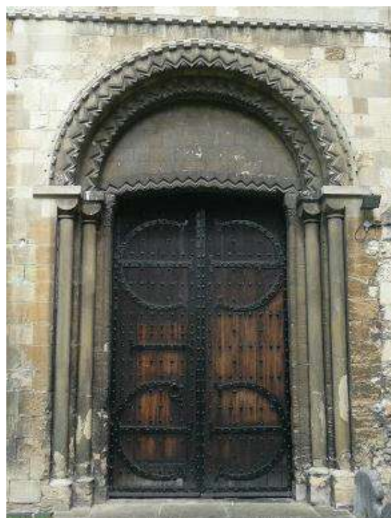
Norman south door featuring a pair of substantial timber doors with large iron strap hinges set in a Norman arch, Abbey Church (EFDC)
