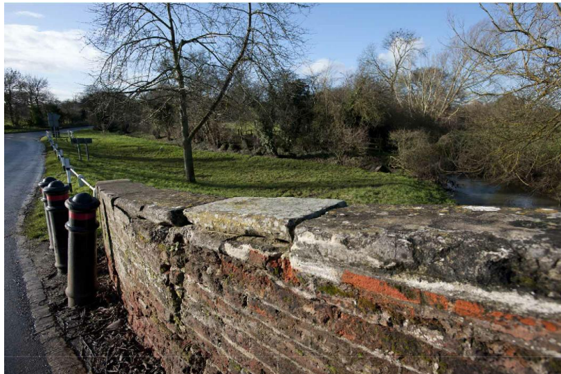
Parapet & Brickwork Damage
