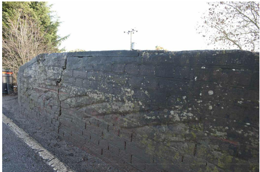
Crack & scoring caused by lorry wheel nuts
