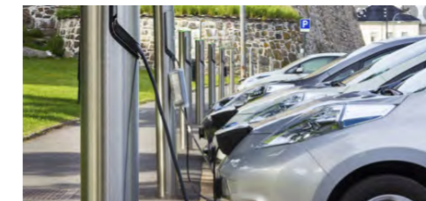
Electric Vehicle Charging Point
