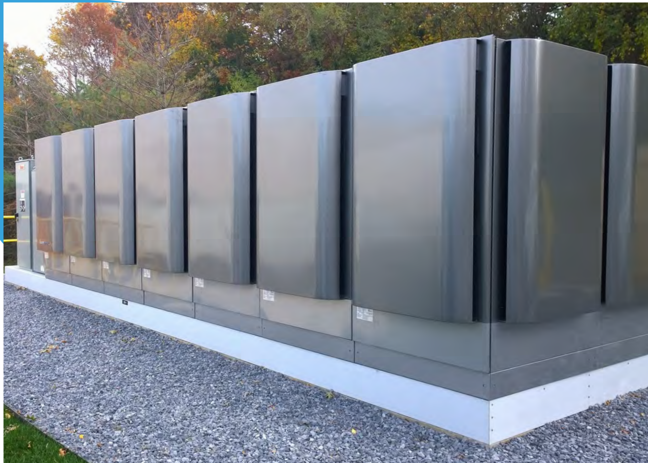
Example Fuel Cell Storage Structure
