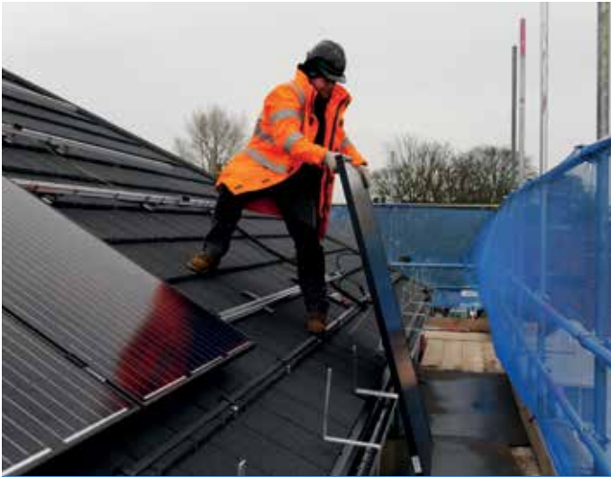
Sustainable energy solar panels
