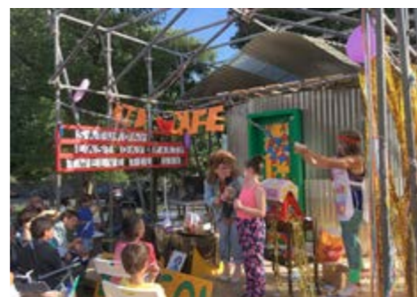
The Portland Inn (Baxendale Studio) A commission to design a building that will host a diverse cultural programme. Part of the brief was that the local community would be able to participate in its construction.
