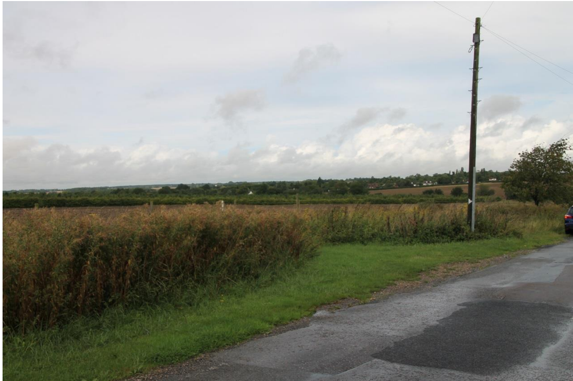
Figure 6 - Shows area of damage to the surface and edges from traffic and agriculture up to the edge of the lane (EPFLane 11)
